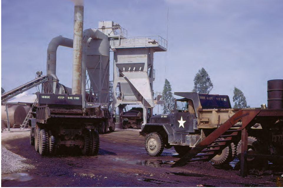
RMK-BRJ industrial sites such as the Phu Cat quarry and asphalt plant provided rock and asphalt for the highway program.
